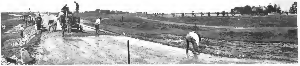
That Stage of the Work Just Preceding the Top Dressing and the Steam Roller which Finishes the Surface.
